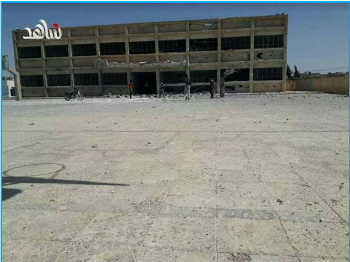
The destruction in the aftermath of a bombing by Syrian regime forces on a school housing IDPs in Tafas city, Daraa – June 14, 2017
