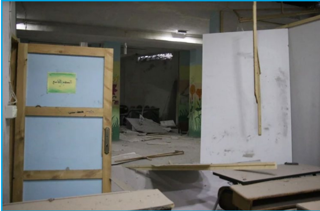
Damages in Sanabel al Festat School in the aftermath of a bombing by Syrian regime warplanes, Hamouriya town – December 3, 2017
