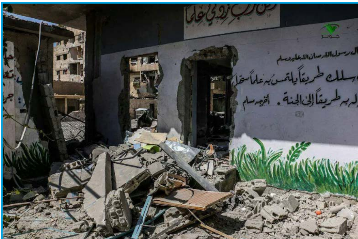
The destruction in the aftermath of a bombing on Tawq al Hamam Orphanage in Jobar neighborhood, Damascus by Syrian regime forces – August 6, 2017
