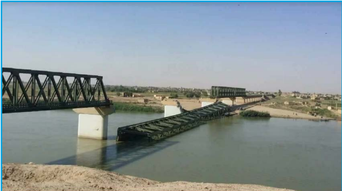
The destruction resulting from a bombing on al Hadid Bridge in al Bokamal city, Deir Ez-Zour by international coalition forces – August 28, 2017
