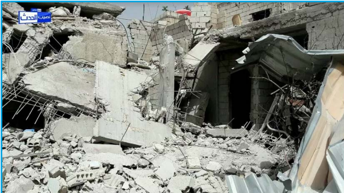
Picture showing the destruction in the residential houses in Nasib village, eastern suburbs of Daraa, after Syrian regime helicopters dropped a number of barrel bombs on them – Sunday, April 30, 2017
