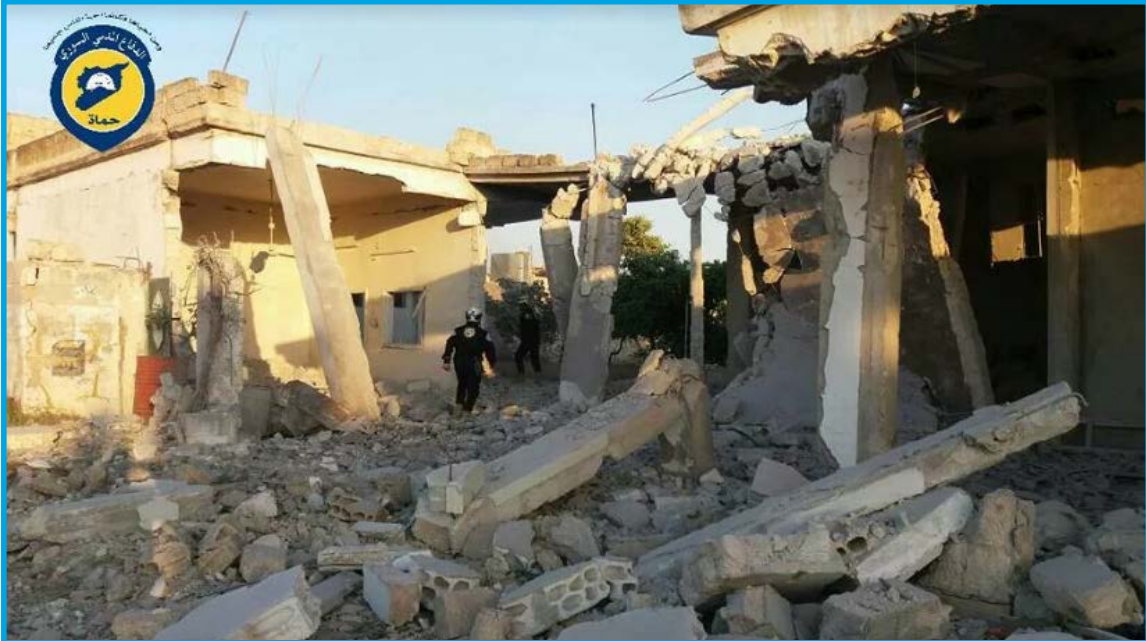
Picture showing the destruction in a house in Kafr Zita city, northern suburbs of Hama, after Syrian regime helicopters dropped a number of barrel bombs on it – Tuesday, April 25, 2017
